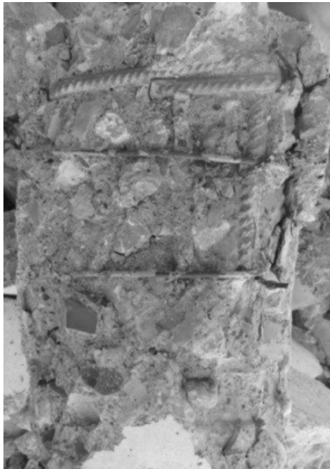
Figure 5. The fracture mechanism of the corroded reinforced rectangular specimens [26]
