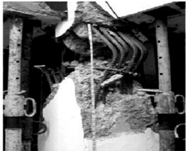
Figure 2. The severe failure in the column due to large distances of transverse reinforcements [6]
